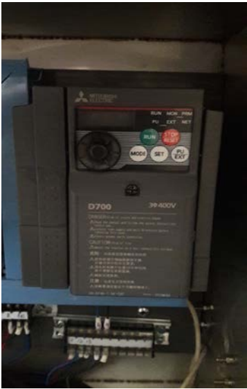
Inverter / VFD Unit – Mitsubishi, Japan
