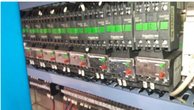
Electrical Component – Schneider, France
